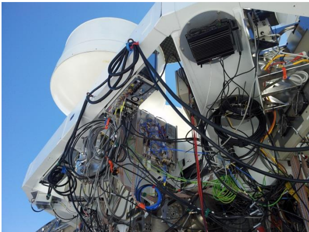
Fig. 10. Prototype digital correlator deployed on the AMiBA site
