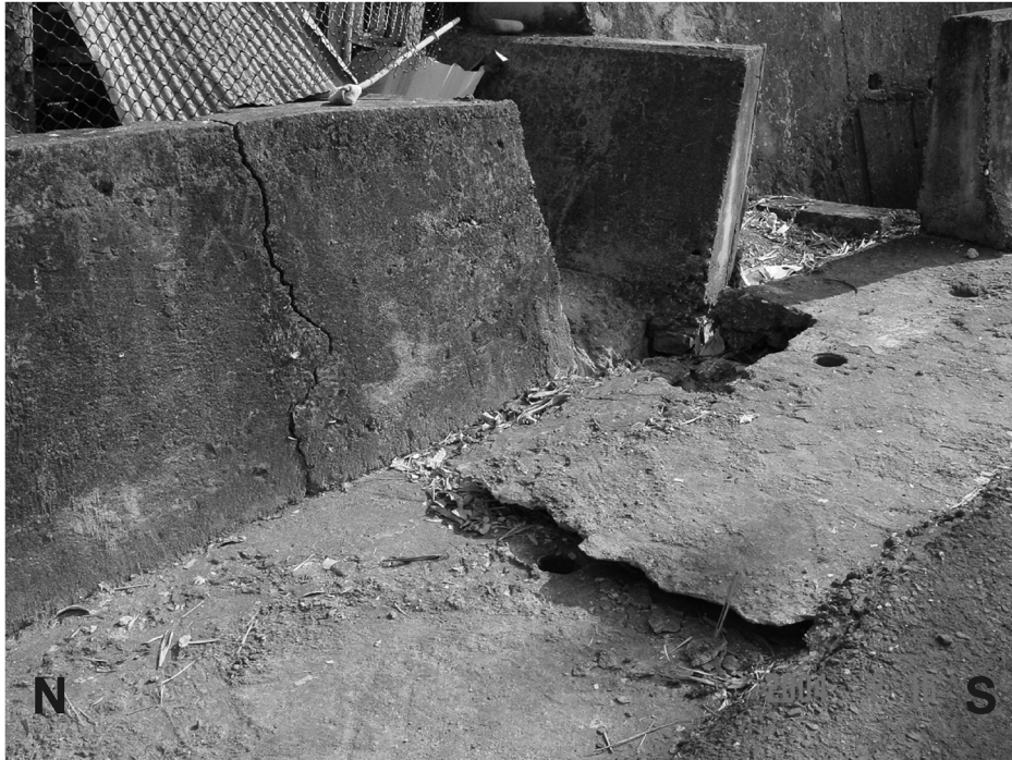
a Compression fractures due to 2003 earthquake at the Tapo slope site
