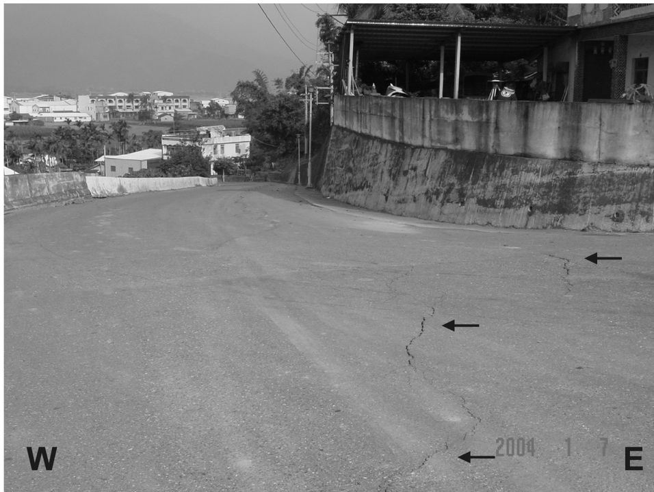
b Transtension fractures due to 2003 earthquake at the Tapo slope site
