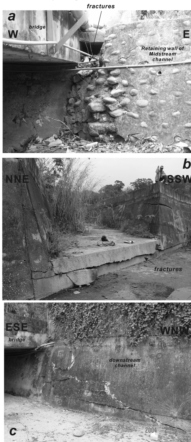
Figure 7. Photographs of surface fractures of the 2003 earthquake on concrete retaining walls and water channels at the Nanhai channel site. (a) Fractures (preexisting) between bridge and midstream water channel. (b) Fractures (preexisting) at the western end of the downstream water channel, (c) Fractures (newly formed) between the bridge and downstream water channel. Circles on the wall mark the locations of nails for measurements of offsets. Note that the fractures usually occurred around the joints between two civil constructions.
