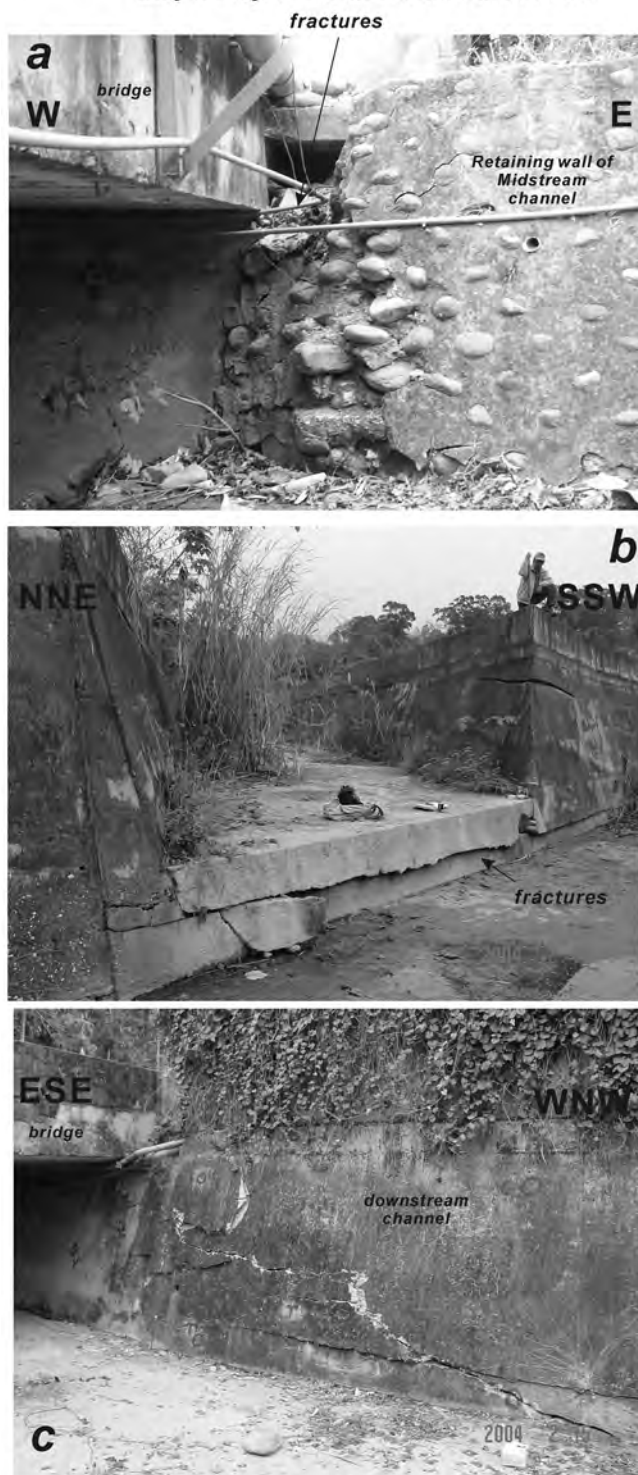
Figure 7. Photographs of surface fractures of the 2003 earthquake on concrete retaining walls and water channels at the Nanhai channel site. (a) Fractures (preexisting) between bridge and midstream water channel. (b) Fractures (preexisting) at the western end of the downstream water channel, (c) Fractures (newly formed) between the bridge and downstream water channel. Circles on the wall mark the locations of nails for measurements of offsets. Note that the fractures usually occurred around the joints between two civil constructions.
