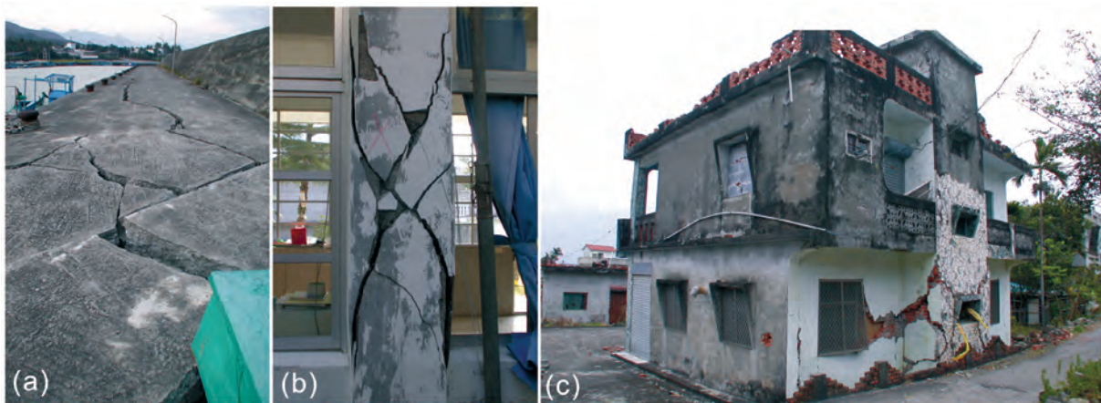
Fig. 2. Damage of human structure resulting from Chengkung earthquake in December 2003 near the epicenter area: (a) Fractures of cemented ground in a small harbor of Hsiao-Gang, about 8 km north of Chengkung. (b) Conjugate fractures in a concrete pillar of the Taiyuan junior high school. (c) Conjugate fractures in the wall of a house in Hsingchang village about 29 km south of Chengkung. See locations in Fig. 1c. These fractures of the concrete structures are interpreted to be mostly resulted from severe ground shaking near the epicenter during the main shock.
