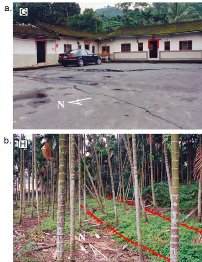
Figure 5. Geological features in the footwall induced by Chi-Chi earthquake faulting. (a) Two fractures and flexures appeared in the courtyard of a house (location G, Figure 2). The amount of uplift by thrusting in the pavement was on the order of 20 to 40 cm. (b) Northeast view of an anticlinal dome (location H, Figure 2). The betel-nut trees were inclined in an opposite direction on the either limb of the dome. The toes of the anticlinal dome are highlighted in red with tip marks, which indicate the down-thrown side.
