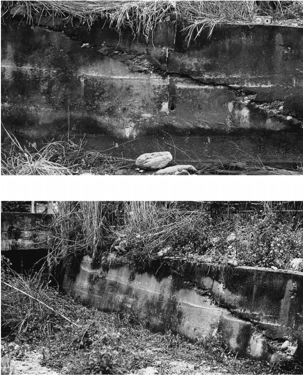
Fig. 8. Example of wall affected by active reverse fault, at the site between Tapo and Chinyuan (channel built in 1987–1990). Southern side of channel (wall striking WNW–ESE, facing north and 1.5 m high). WNW on right. Location in Figs. 2 and 3. Above (a): fault in 1992 (observation on 24-01-1992, ref. 2199). Below (b): fault in 1994 (observation on 30-01-1994, ref. 2828). From 1992 to 1994, horizontal shortening of 5.1 cm occurred, nearly parallel to wall strike. See also Tables 1 and 5.
