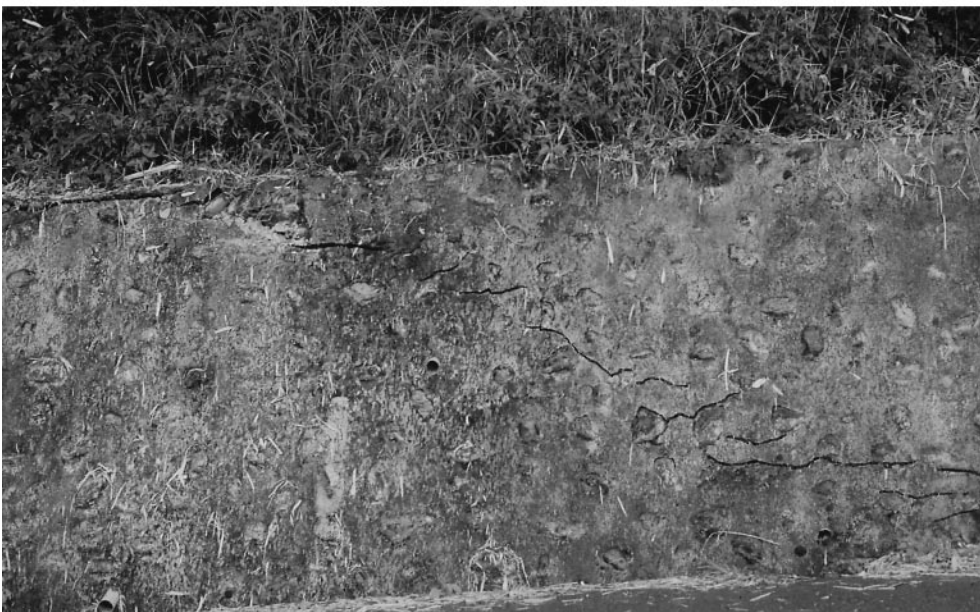
Fig. 4. The evolution of the Chihshang Fault until 1986, as recorded by two walls successively built across the active fault scarp, at the southwestern entrance of Tapo Village (location in Figs. 2 and 3b). Wall strikes NNW–SSE and faces west. See also Tables 1 and 2. Above (a): the faulted wall in 1982 (observation on 19-12-1982, ref. 188). Date of wall construction unknown. Scale: Chu Hao-Tsu. Below (b): same location, en-échelon fractures indicating ongoing reverse shear in new, higher wall (observation on 21-11-1986, ref. 637). Date of construction of new wall: early 1984. This fault is the upper fault of Tables 1–6 and Fig. 6. Wall height: 1.8–1.85 m. SSE on right.
