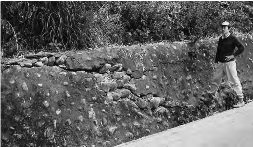
Fig. 5. The 1990–1992 evolution of the Chihshang Fault recorded by a wall across the active reverse fault scarp, at the southwestern entrance of Tapo village (location in Figs. 2 and 3b). Same place and wall as for Fig. 4b (built in early 1984, striking NNW–SSE, facing west and 1.8–1.85 m high). SSE on right. Note increasing damage along reverse fault. Between (a) and (b), horizontal shortening of 2.2 cm has occurred, nearly parallel to wall strike. See also Tables 1 and 2 (the fault is the upper fault). Above (a): faulted wall in 1990 (observation on 19-01-1990, ref. 1532). Scale: Lee Teh-Quei. Below (b): same faulted wall in 1992 (observation on 23-01-1992, ref. 2137). Scale: Chu Hao-Tsu.
