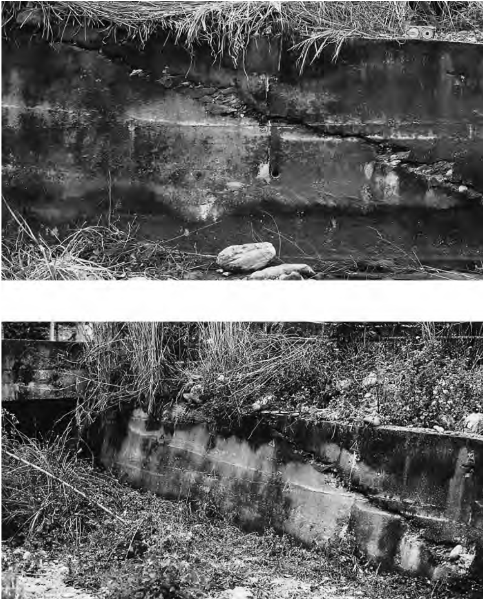
Fig. 8. Example of wall affected by active reverse fault, at the site between Tapo and Chinyuan (channel built in 1987–1990). Southern side of channel (wall striking WNW–ESE, facing north and 1.5 m high). WNW on right. Location in Figs. 2 and 3. Above (a): fault in 1992 (observation on 24-01-1992, ref. 2199). Below (b): fault in 1994 (observation on 30-01-1994, ref. 2828). From 1992 to 1994, horizontal shortening of 5.1 cm occurred, nearly parallel to wall strike. See also Tables 1 and 5.
