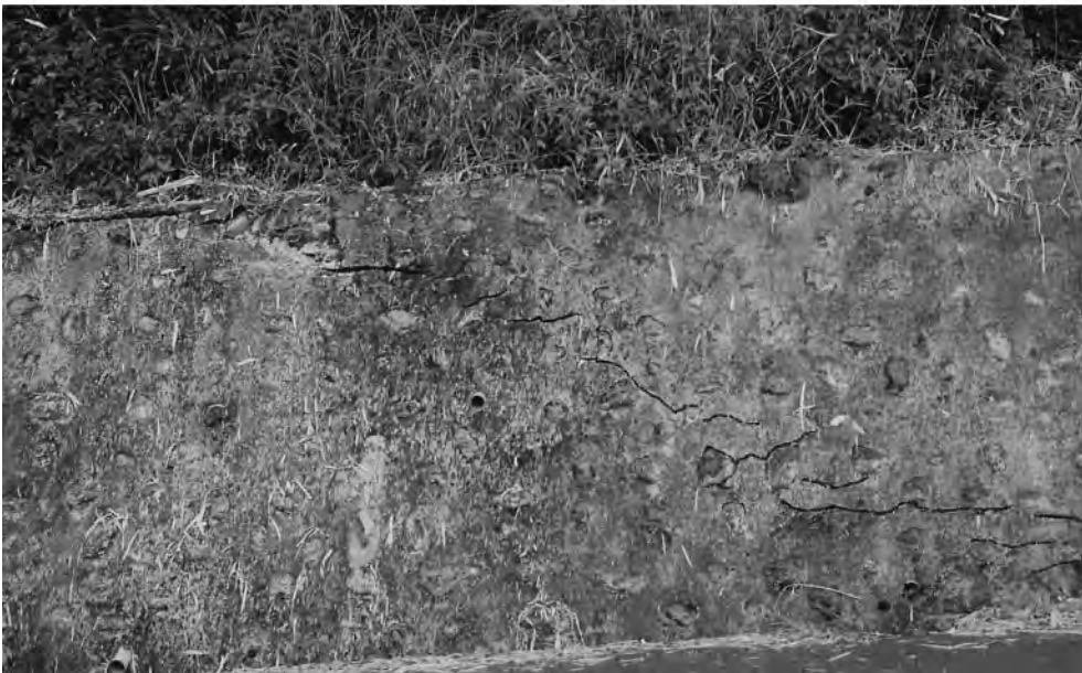
Fig. 4. The evolution of the Chihshang Fault until 1986, as recorded by two walls successively built across the active fault scarp, at the southwestern entrance of Tapo Village (location in Figs. 2 and 3b). Wall strikes NNW–SSE and faces west. See also Tables 1 and 2. Above (a): the faulted wall in 1982 (observation on 19-12-1982, ref. 188). Date of wall construction unknown. Scale: Chu Hao-Tsu. Below (b): same location, en-échelon fractures indicating ongoing reverse shear in new, higher wall (observation on 21-11-1986, ref. 637). Date of construction of new wall: early 1984. This fault is the upper fault of Tables 1–6 and Fig. 6. Wall height: 1.8–1.85 m. SSE on right.
